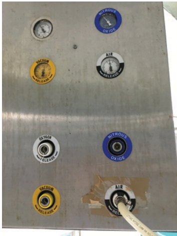
Figure 1: Oxygen pipeline connected to air accidentally; leading to the mishap!
