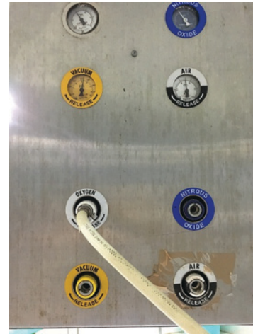
Figure 2: DISS and correct approximation of oxygen pipeline to its port on pendant.
