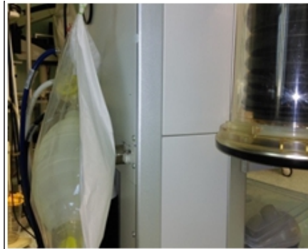
Figure 2: AMBU bag obstructing the scavenging
